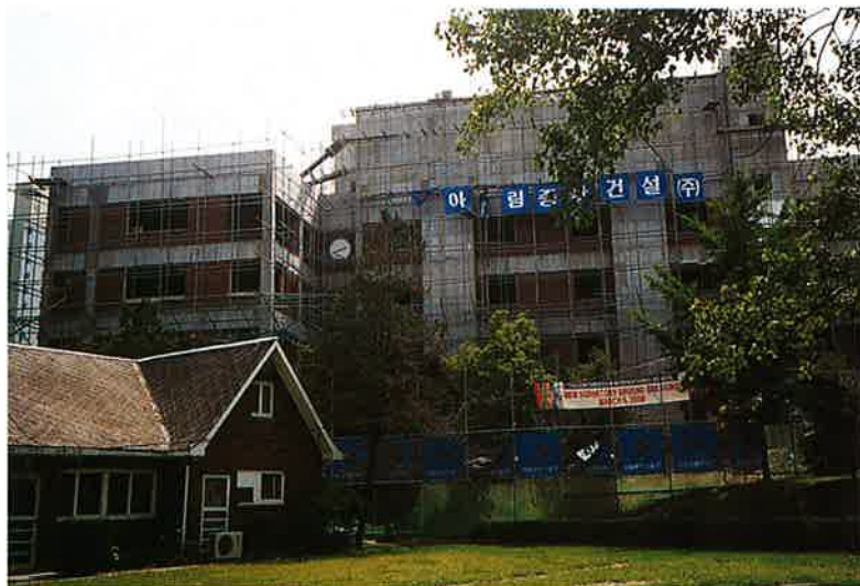
New four-story on-campus dormitory under construction as viewed from the quad in front of the teacher duplex
